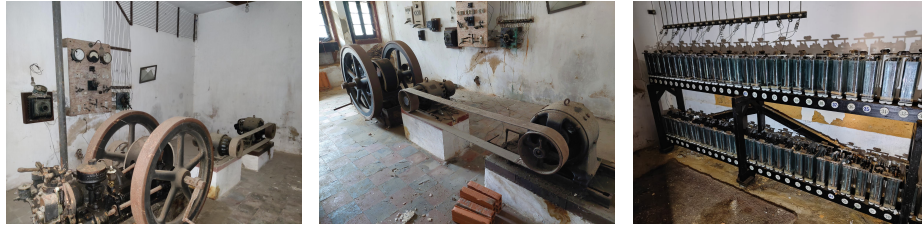
(a) Left view of the machine (b) Right view of the machine room. (c) Tudor battery rack.
